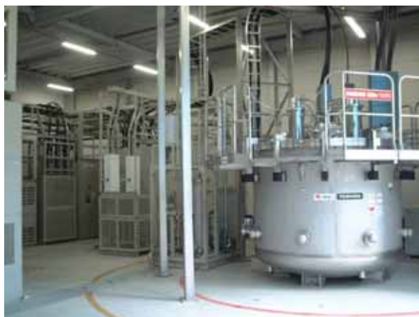
Fig.3 An External View of a Superconducting Coil System
