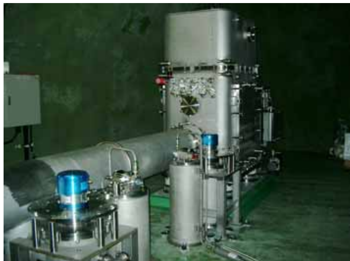
The 4-K and 80-K low-vibration pulse tube refrigerating systems for cooling a gravity wave detection mirror installed in the ground of Kamioka Mine.
