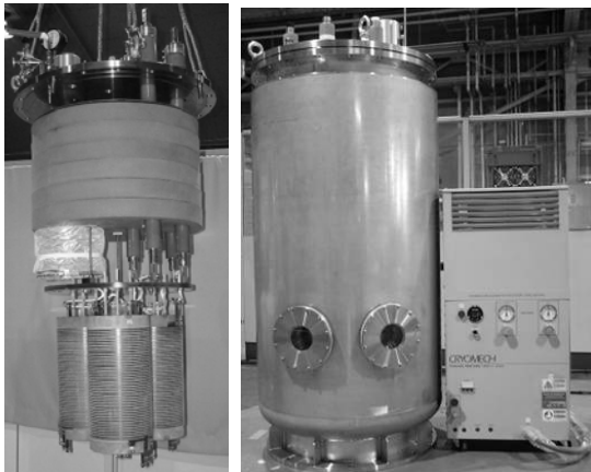
Fig. 1 Three-phase current limiting coils (left), Subcooling liquid nitrogen vessel and cryocooler compressor (right)
