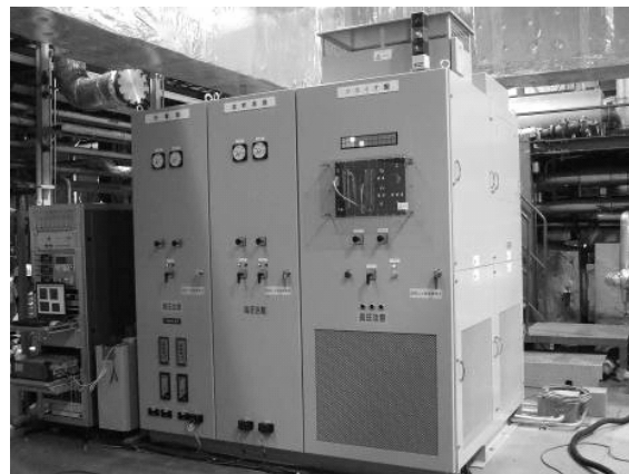
Fig. 2 Current limiter panel (consists of a receiving panel, circuit breaker panel, and a cryopanel)
