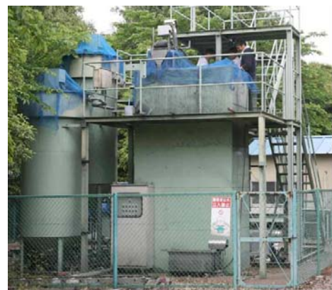
Fig. 1 Magnetic Activated Sludge Process Pilot Plant — The sewage of 50 people can be treated without generating excess sludge.
